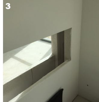
3 The fireplace wall is not secured against false draft in the sides.
